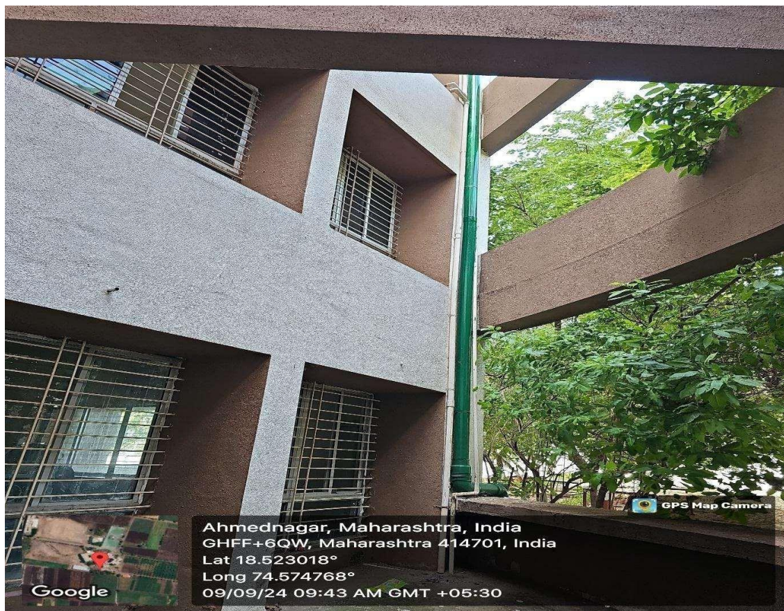
Green pipe indicate rain water harvesting system
